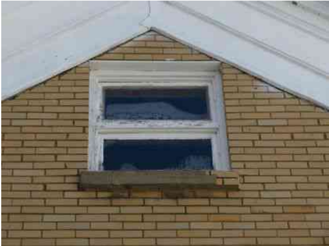
Photo 10.4: Detail of gable window at west elevation. Note deteriorated and poorly patched brick sill.
