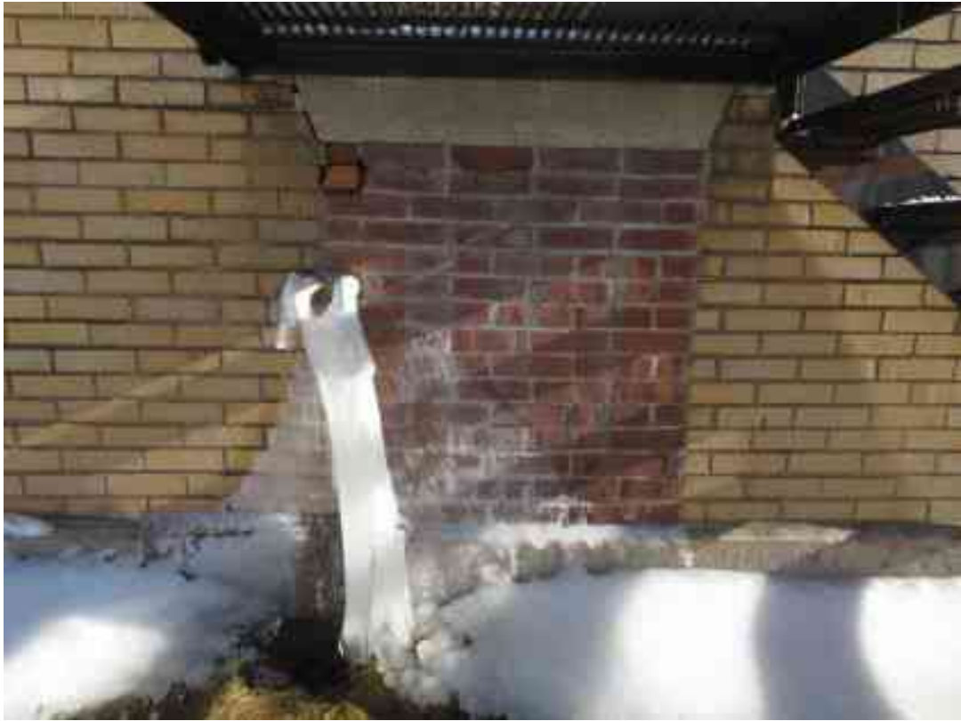
Photo 10.3: Detail of frozen basement sump pump discharge to exterior at Southwest Exit.
