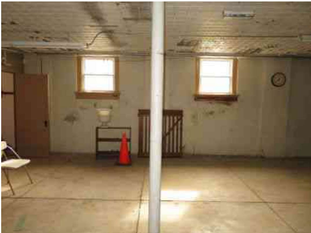
Photo 34: (below) Looking south in Center Basement. Note tin ceiling and water damage below windows.
