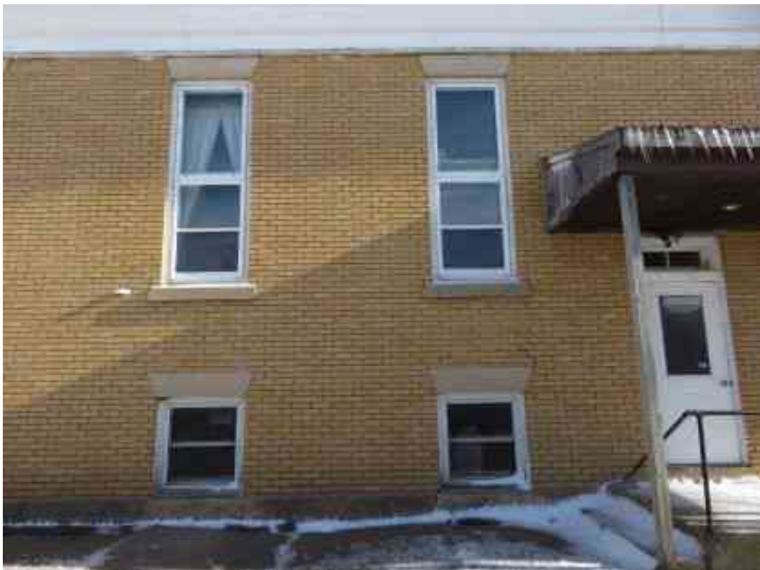
Photo 10.2: (below) Detail of exterior, south face. Note miscellaneous step cracks above the basement windows.
