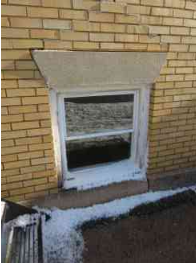
Photo 10.7: Detail of displaced lintel at basement window with triangular step-cracking above it.
