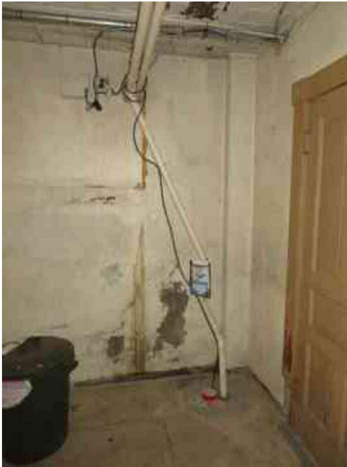
Photo 35: (left) Detail of sump, pump, and discharge piping at southwest corner of Center Basement.
