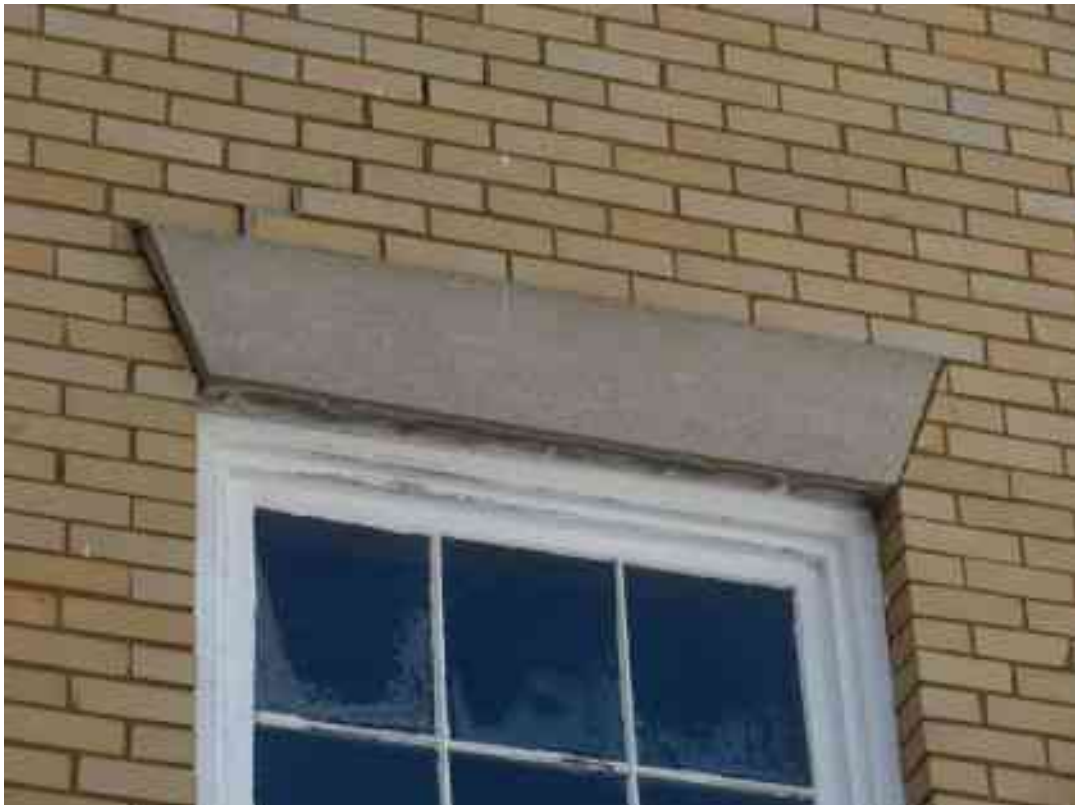
Photo 10.6: (below) Detail of displaced header and step cracking at typical window.
